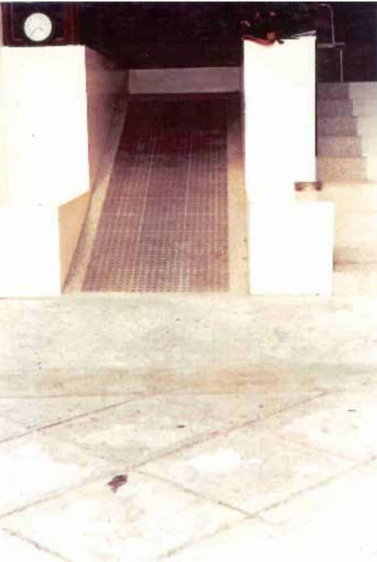
Illustration 17 A steep and straight ramp, but with no handrails. Slope gradient of the ramp is equal to the run of the 10 steps.
