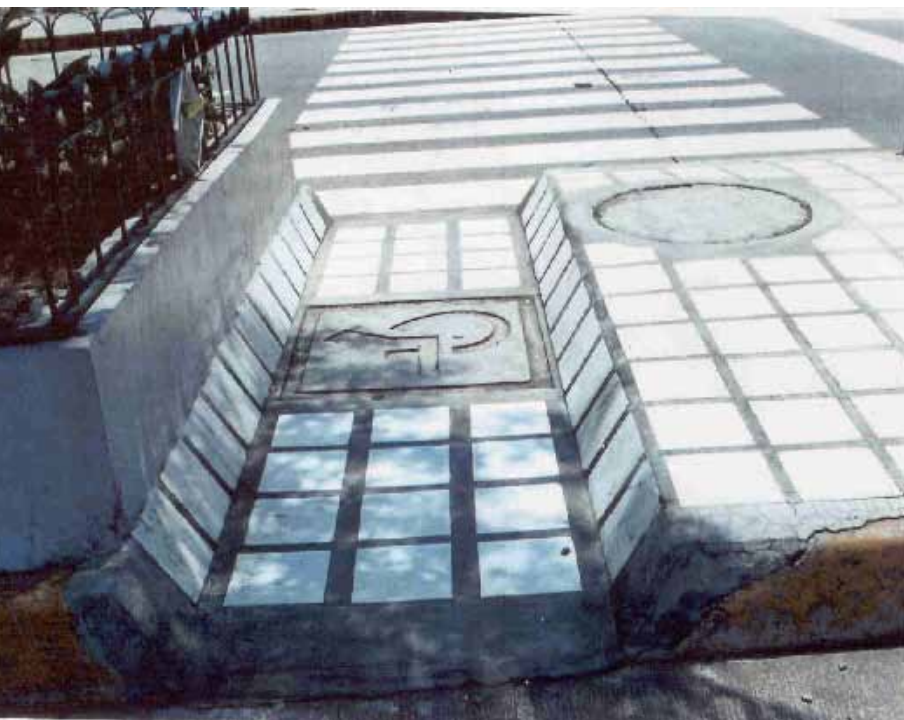
Illustration 18 A curved cut out with UN symbol of accessibility on the pavement. Major sidewalks of Metro Manila have been retrofitted by the DPWH to accommodate wheelchair user.
