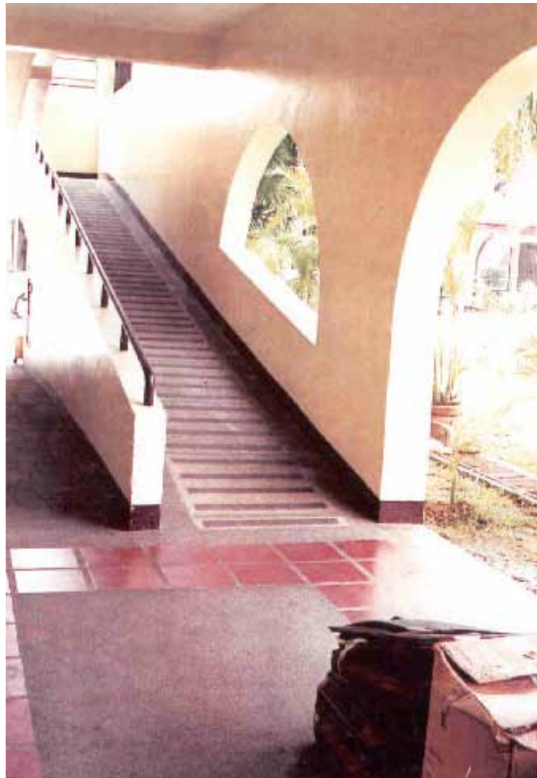
Illustration 18 A long, straight and steep ramp, leading to the main entrance of a resort establishment. The slope gradient is about 1 is to 4.
