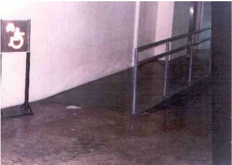
Illustration 22 A ramp with conforming ramp gradient, and complying handrails. In addition, there is a signage which states that the ramp is for the wheelchair user.
