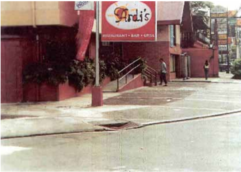
Illustration 15 A steep ramp with 2-level handrail on one side. The slope gradient of the ramp is equal to the run of the 5 steps.
