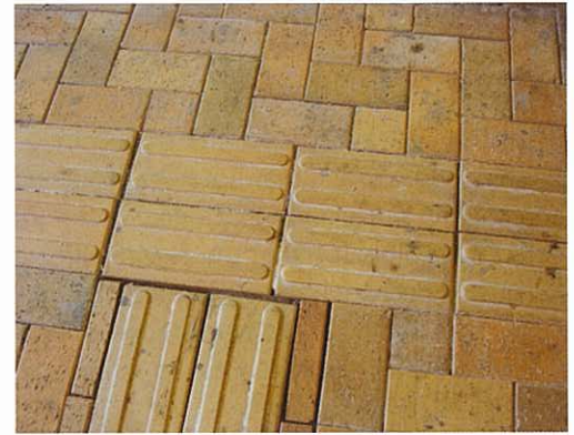
Tactile paver in same colour as the surrounding tiles is not distinguishable by the visual impaired but increasing chances for trip over.
