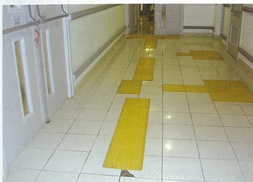
PVC tactile paver can be peeled off leaving disjointed guide path leading to nowhere but confusion.
