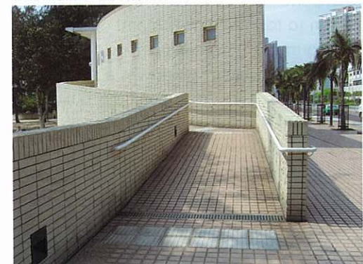
Fig 5. Provide ramp with continuous handrails on both sides. The addition of a low level handrail would facilitate access by younger children and wheelchair users.
